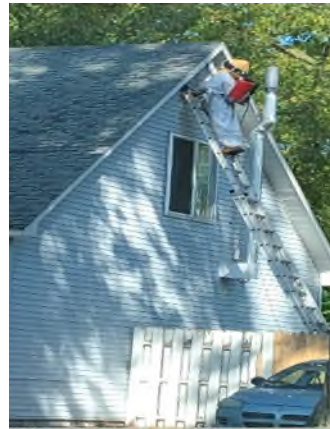
34682 Beacon removal of hornet nest
