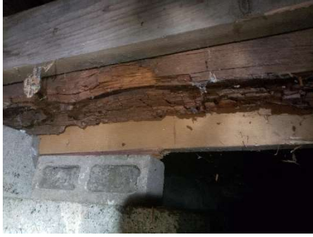
34450 Capitol dry rotted support beam
