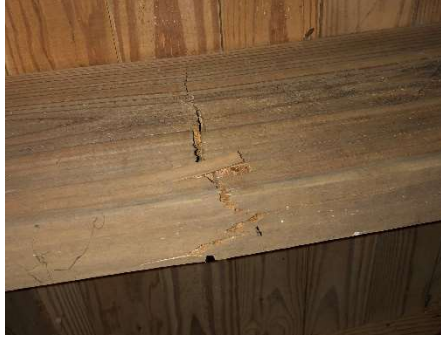
34450 Capitol cracked floor joist
